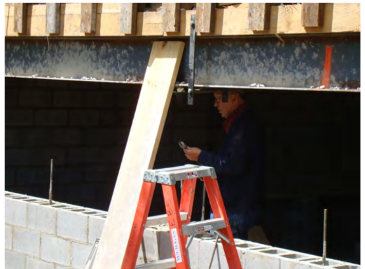
Bob Watros installs Brad Perkins' invention. A roller bar is suspended from the beam in order to facilitate removing the steel beam.
