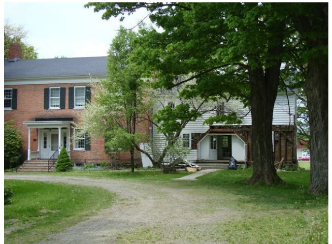
Preparation for sill and foundation work on east wing of Southworth Homestead soon to begin
