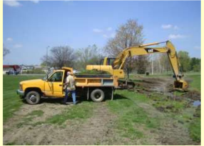
Cooperation in Progress - all donated! Widening the swale between Southworth Homestead and Willowbrook properties Cornell drove the backhoe loaned by Roger Beck which was transported to the site by the town of Dryden. Skeeter Heidt drove the dump truck on loan from Reggie Brown. Bob Watros and the village laid out the site work.
